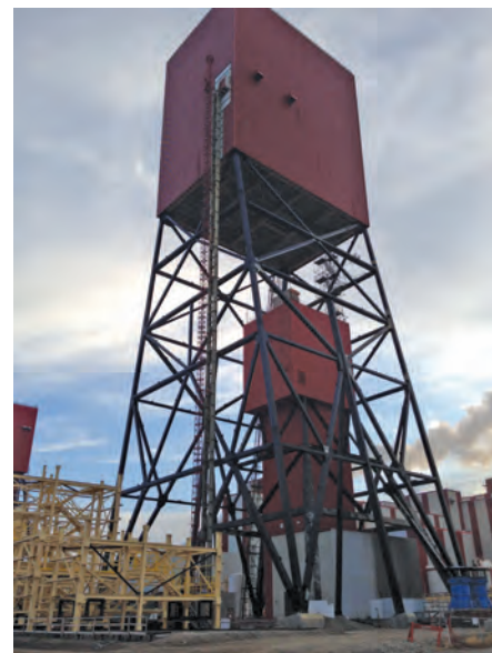
WSP argues that there are numerous factors involved with determining the right conveyance guide system for any operation
