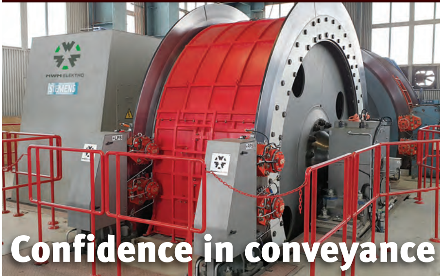
Koepe type 4-rope hoisting machine with direct AC synchronous drive at KGHM's Rudna mine supplied by MWM Elektro
